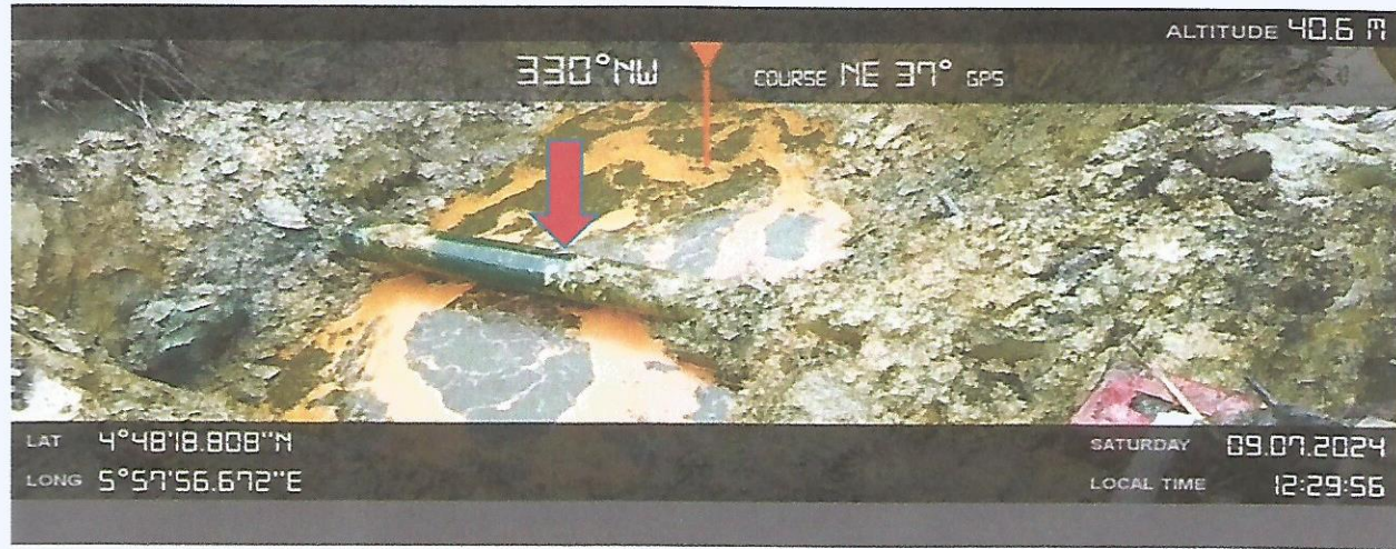
Pic1: Showing pipeline with the leak point at 6 O'clock position
